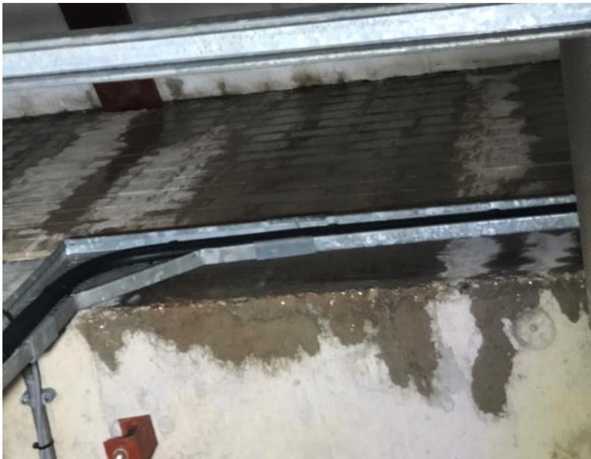
WATER INGRESS DUE TO ROOF LEAKING
